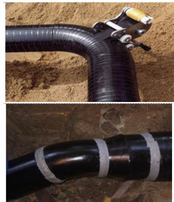
Fig.1. Insulation on bends with PE +BR strips (the one strip system) and compensation for the diameter differences (reductions) (unevenness) with butyl rubber mastic (applicable on tees and tapping tees)
