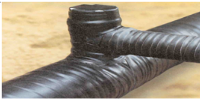
Fig. 4. Tee and tapping tee insulated with PE + BR strips (the two-strip system)
